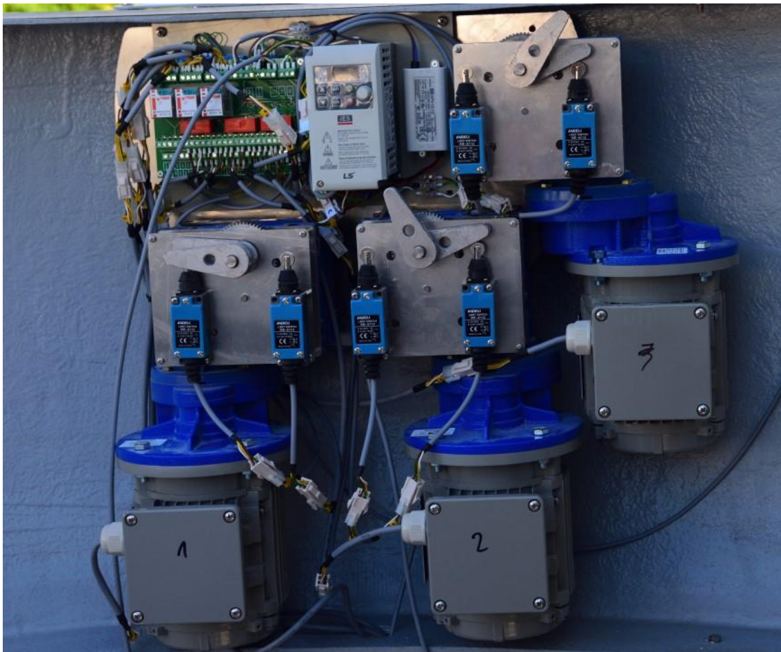
Figure. 72 – View of the limit switches assembly and drive units
