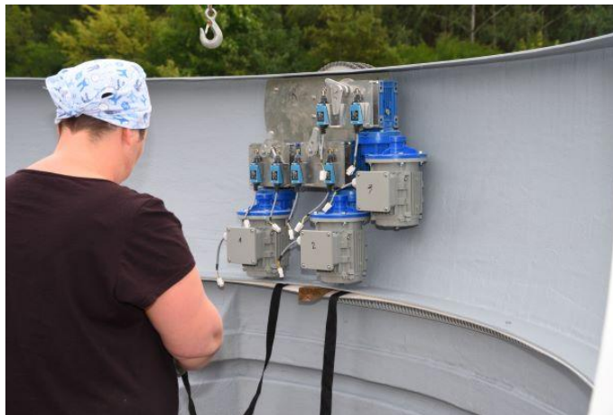
Figure. 6 – putting the transport slings between the top and bottom part of the observatory base
