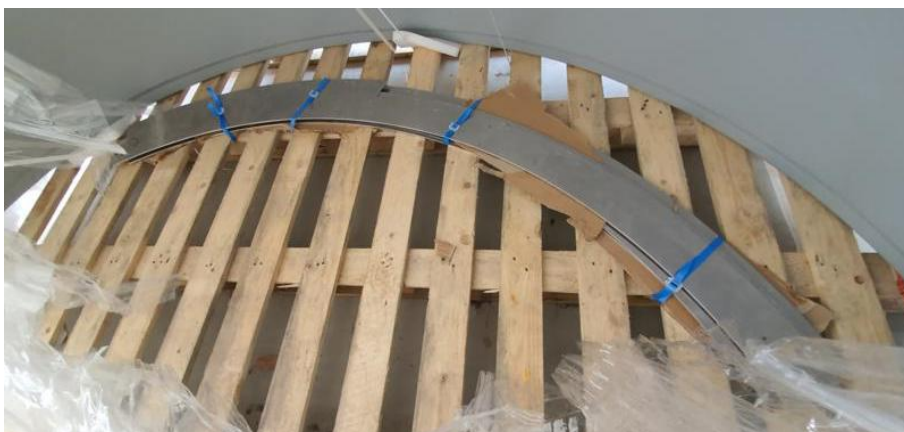
Figure. 3 – elements of the upper ring stiffening the base of the Clamshell observatory
