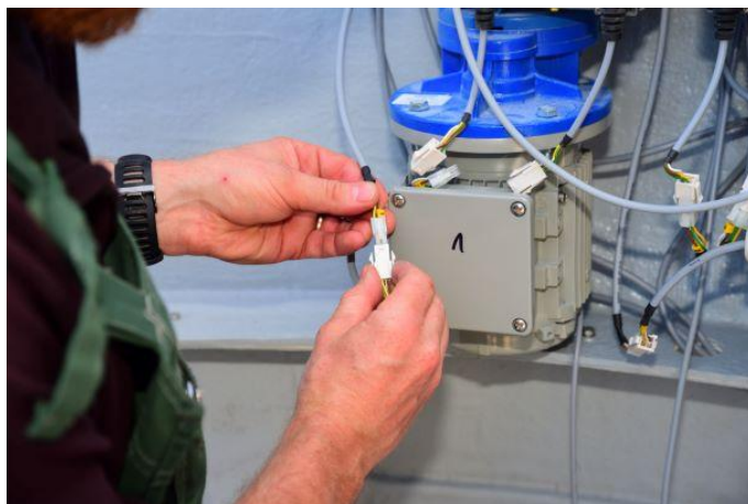
Figure. 33 – connecting the motor power wires on the left side of the observatory base to the controller
