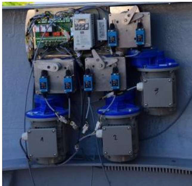
Figure. 35 – view of limit switches and observatory shutters control mechanism
