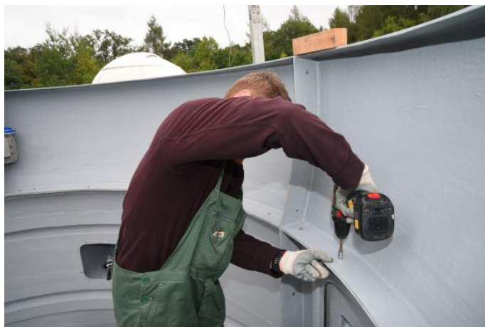
Figure. 25 – Final connection of the upper elements of the observatory base with screws
