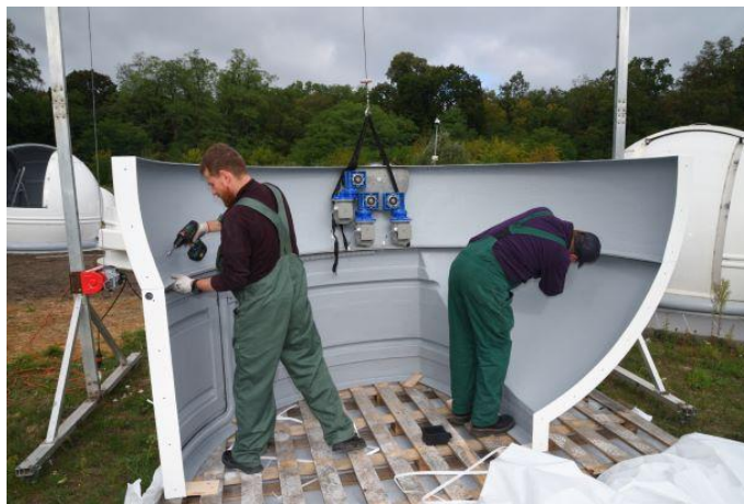
Figure. 7 – dismantling of M6 screws connecting the top and bottom of the observatory base to be transported to the installation site
